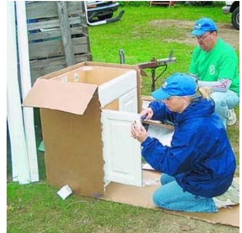
ImageSoft Human Resources Coordinator Leanne Eastmar attaches hardware to a new bathroom vanity while her husband Ken, prepares the plumbing parts. (IMAGESOFT)
